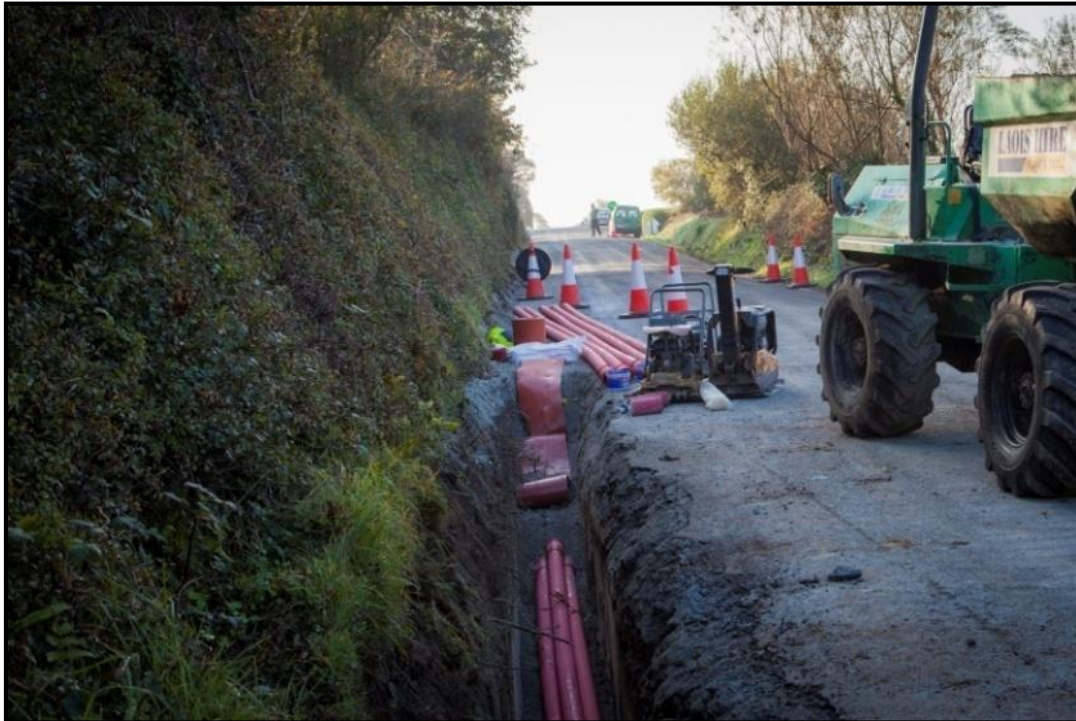
Figure 3-2 Photograph of cables installed in a trench on a public road.
